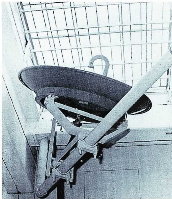
(Inset) Microwave dish for KSD-TV STL is mounted inside the transmitter building, protected by a heavy duty plastic covering and 8-inch steel mesh.
